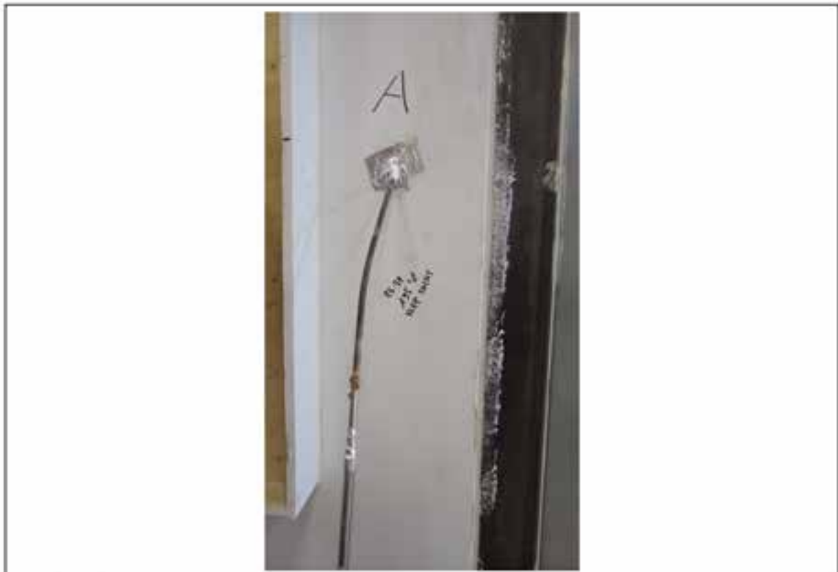
Photo C. 6: Closing time damper B
