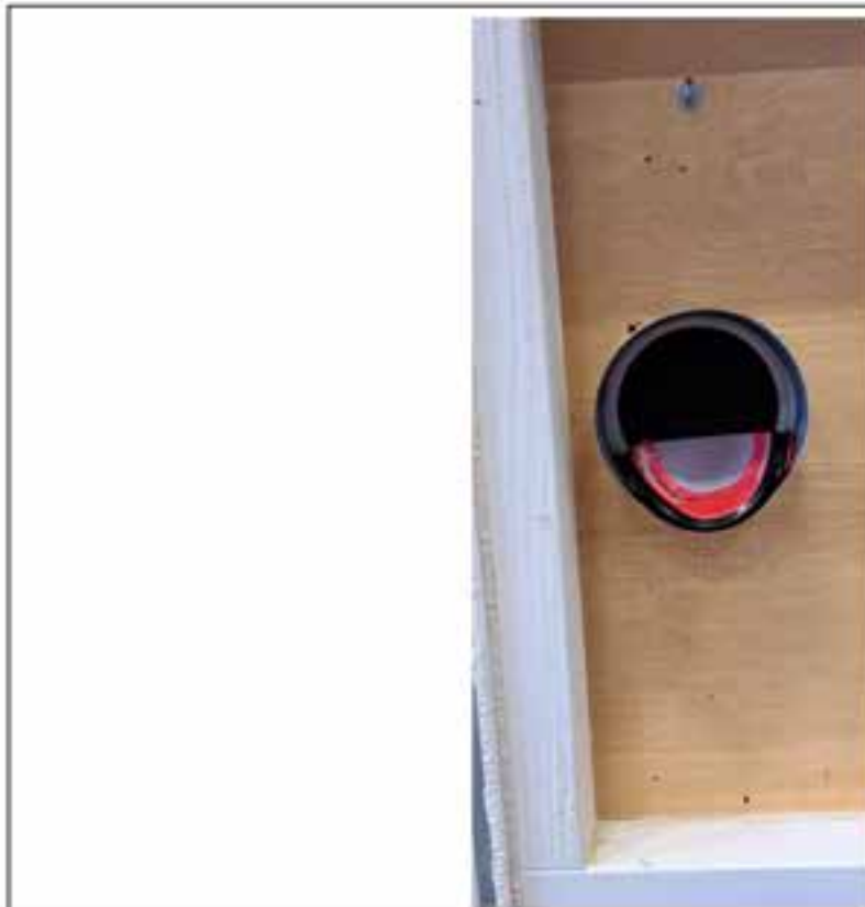
Photo C. 8: Damper B (exposed side)
