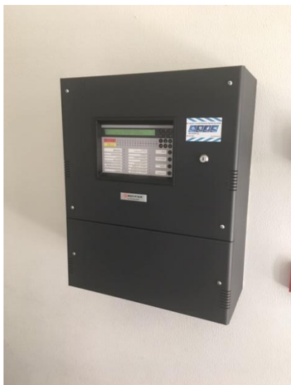
brandmeldcentrale in entree
