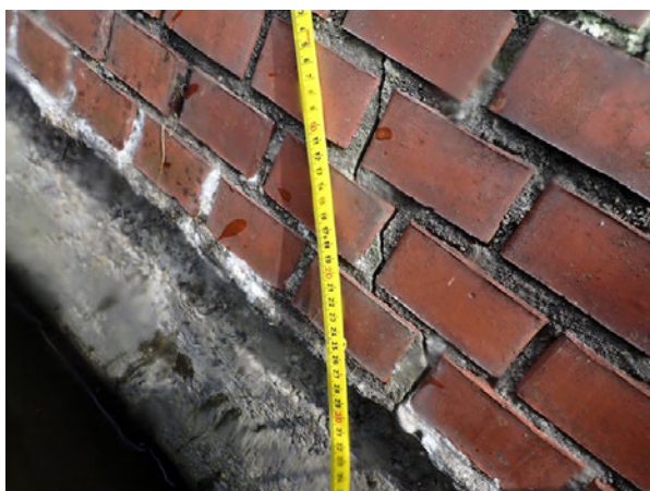
Foto 8.3: Scheur in wand.
