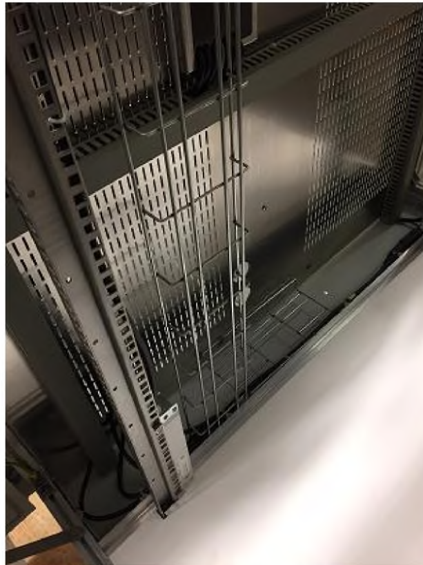
Cable tray : left of 19"compartment
