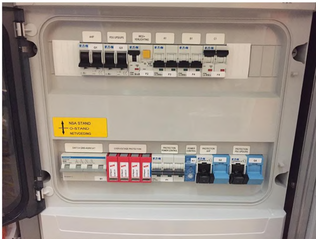
Overview electrical box incl. Components
