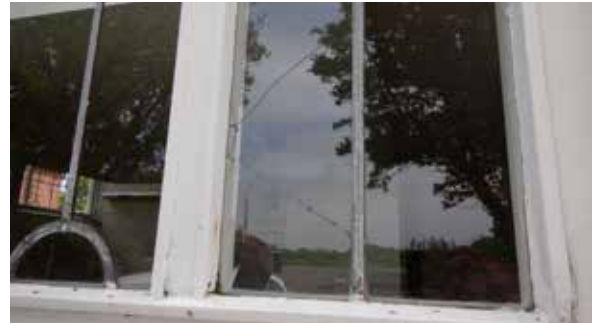
Glasschade in glas in loodraam
